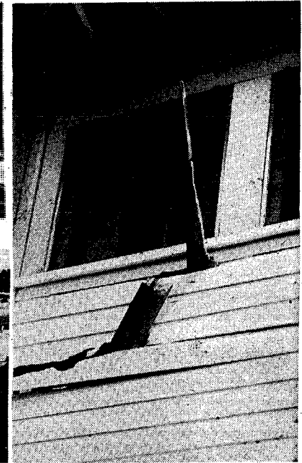
HIGH WINDS DRIVE PLANKS THROUGH WALL. Fort Benning's Officers Quarters Damaged
